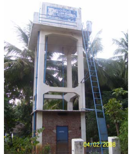
Pappanchalla Overhead Reservoir. Lowest part of the columns supporting the reservoir are joined with brick masonry and enclosed into an office space
